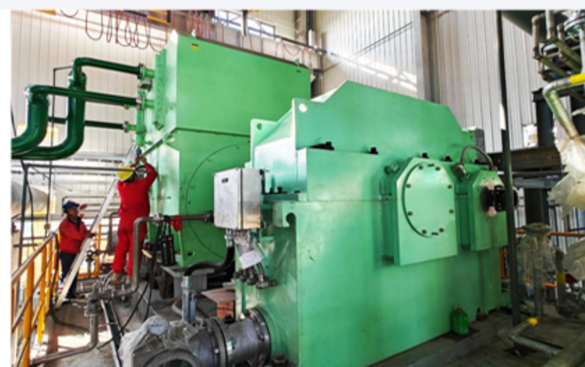
Hydrogen power generation
