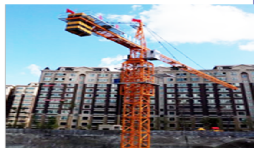
Crane hoist control
