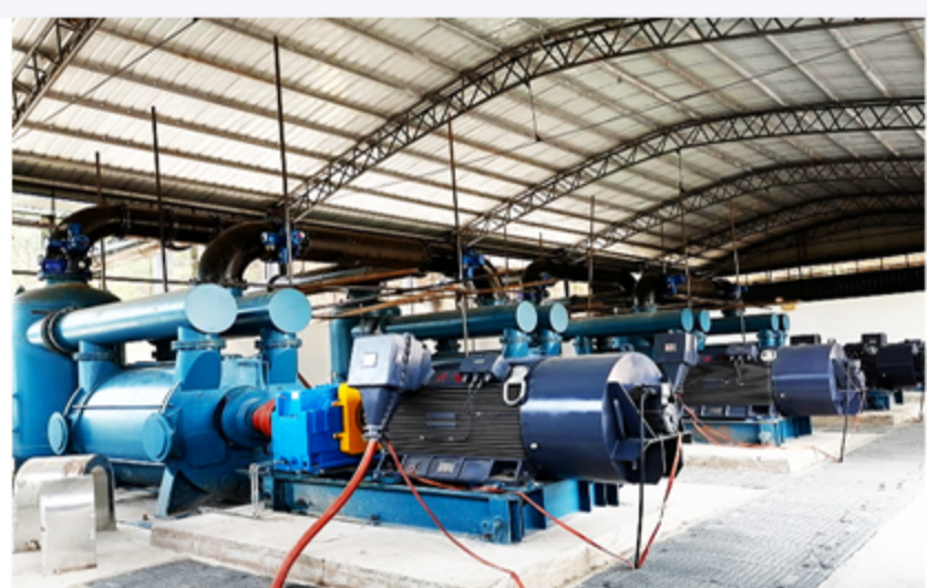
Water pump/water treatment
