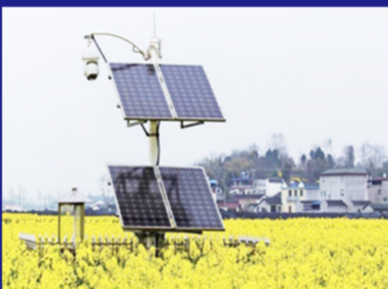
Photovoltaic water pump
